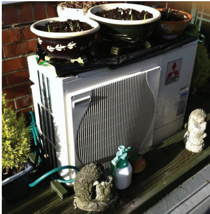
Figure 2. Air source to water heat pump external unit, South Tyneside, showing new elements being fitted into the existing physical external space. This example indicates how integration between the old and the new extends beyond the immediate energy related practices such as heating, washing and ventilation, to other activities such as gardening.
