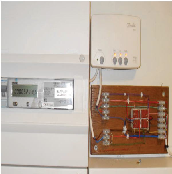
Figure 1. Jens observed that DE often only optimised his heat pump once a day, so he made an electric hob that allowed him to optimise twice a day.
