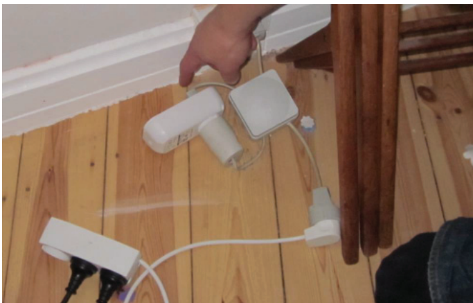
Figure 2. Martin's homemade ground connection for power nodes
