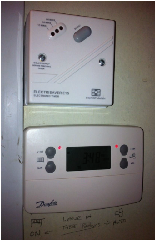
Figure 1(a). Hot water boost (top) and main control with handwritten instruction to leave in set positions (below)
